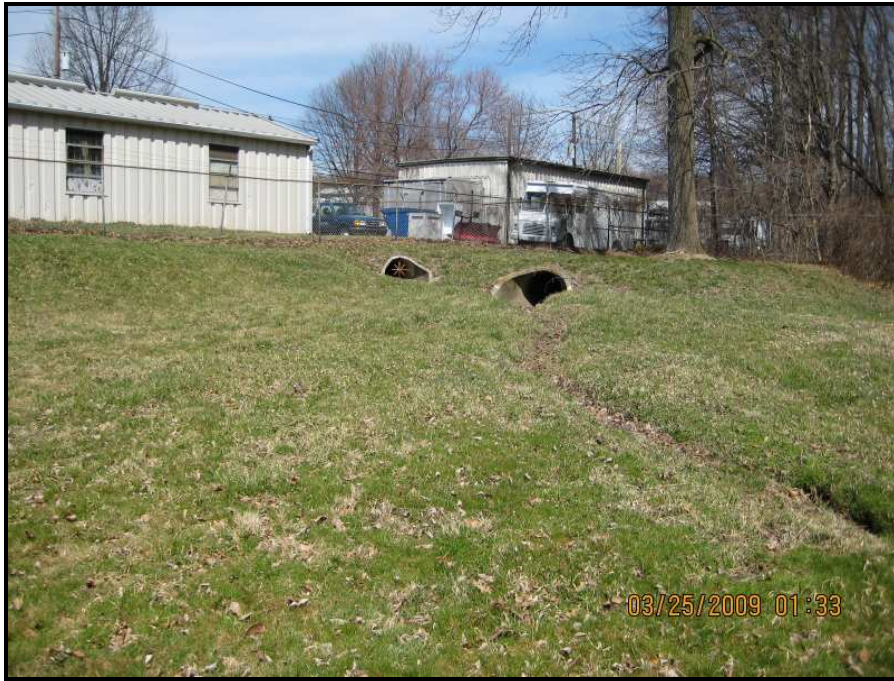
Photo 3 Stormwater Retention Pond Located South of Facilities Maintenance Department Garage
