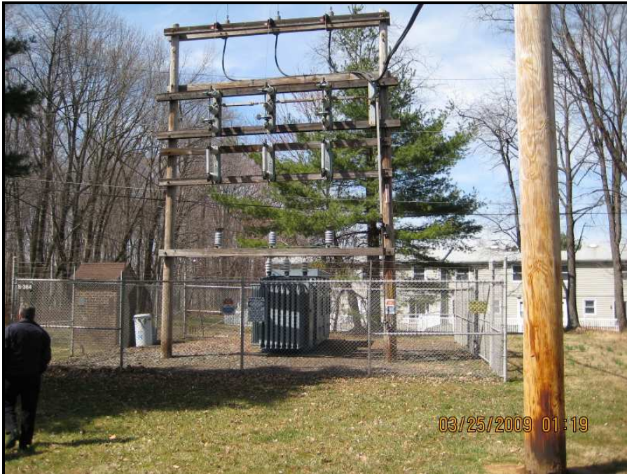
Photo 2 Shenandoah Woods Power Transfer Station
