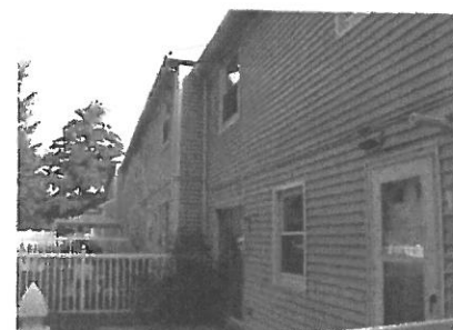
REAR FACADE CONDITION
