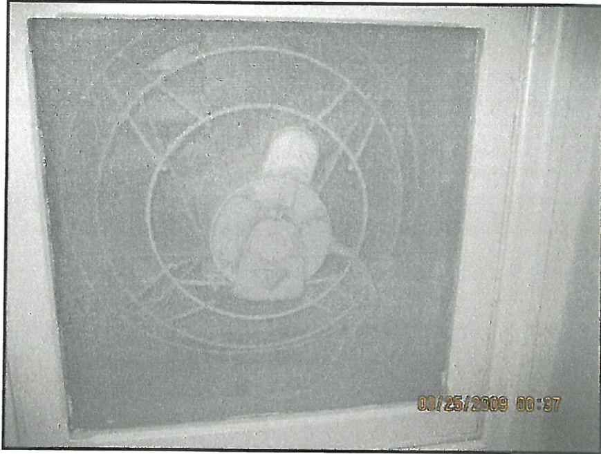
Photo 3 Attic Entrance and Ventilation System
