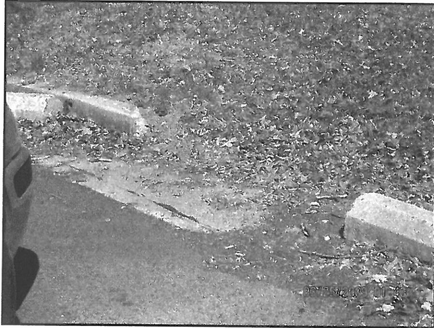
Photo 5 Curbing Removed to Facilitate Drainage During Hurricane Floyd Located on the Northern Portion of the Property Near 403 Skyhawk Drive
