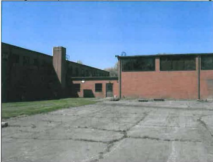
Figure 6. South elevation of the Horsham Memorial USARC, showing rear of the main block, one-story hyphen, and double-height rear wing with clerestory lights for the drill/assembly hall, facing northwest.
