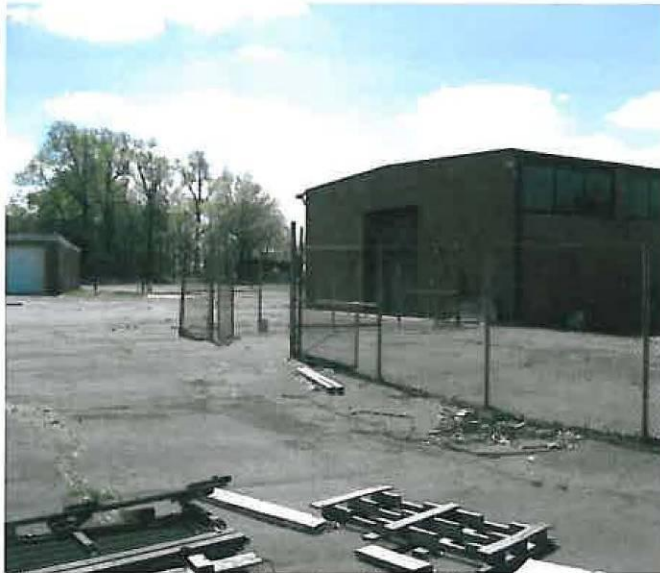
Figure 5. Rear (east) and north elevations of the rear wing (drill/assembly hall), showing the roll up door of the Horsham Memorial USARC, facing southwest
