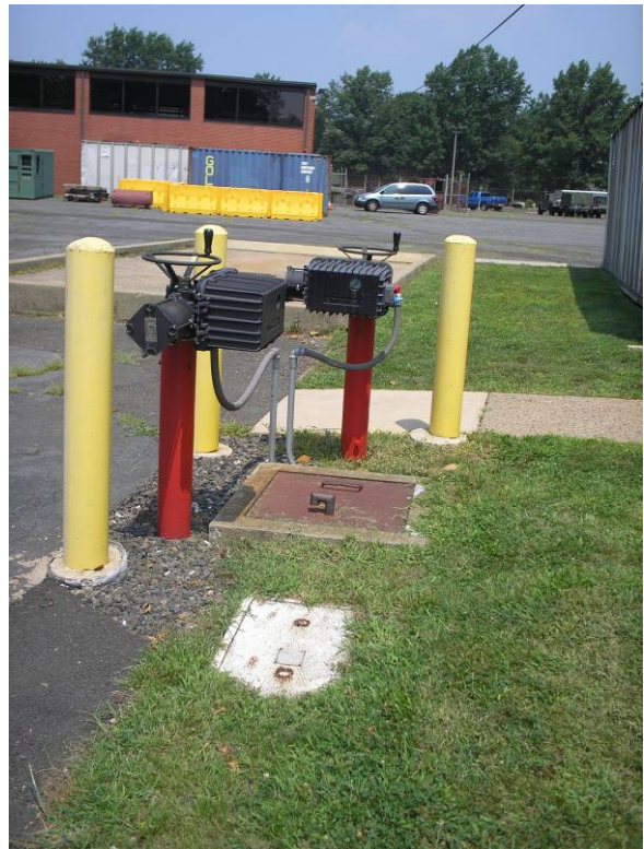
4. Oil/water separator, between wash rack and OMS building.
