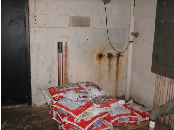
1. Boiler room inside the main building, facing east.
